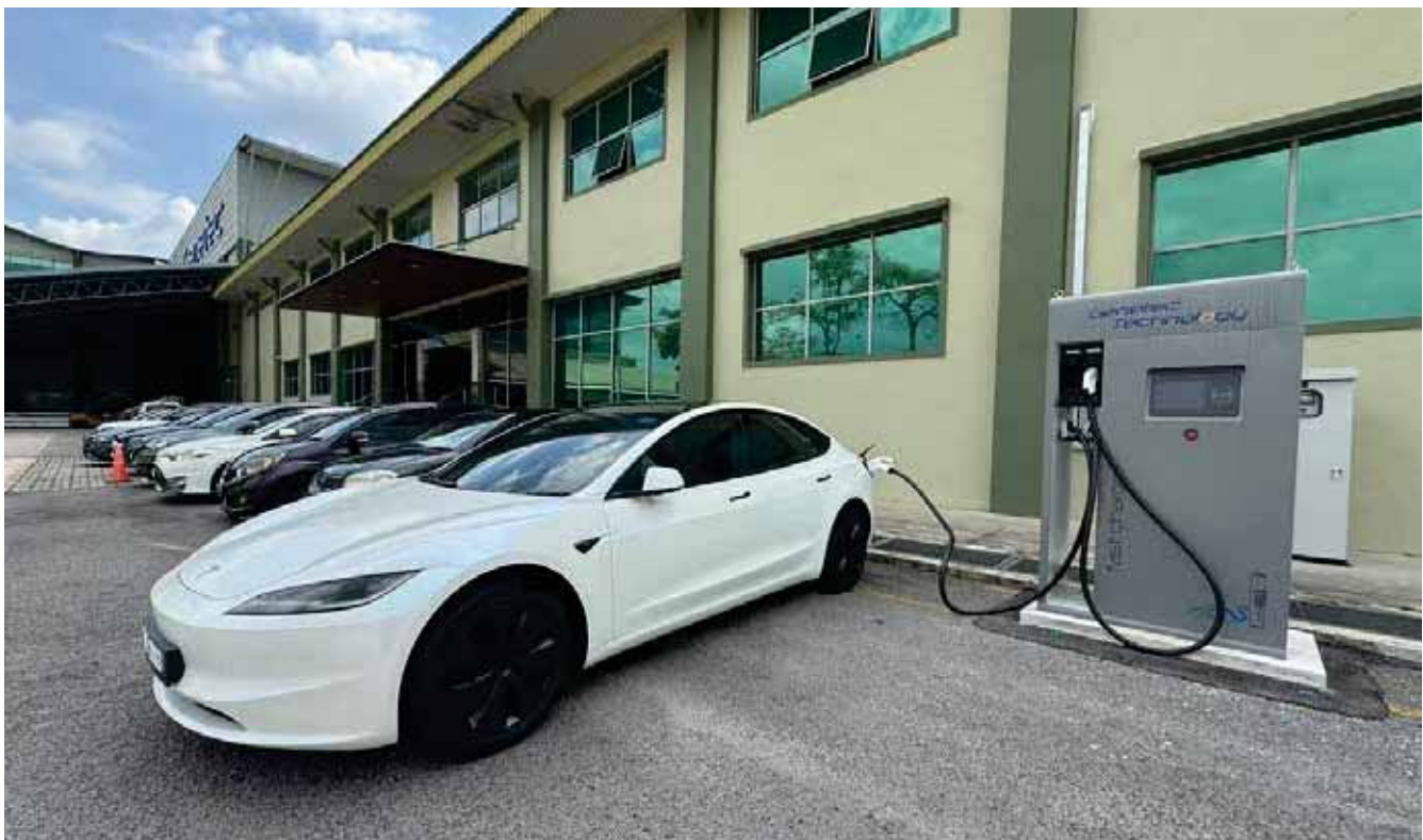
EV Charging Station in EPIC
